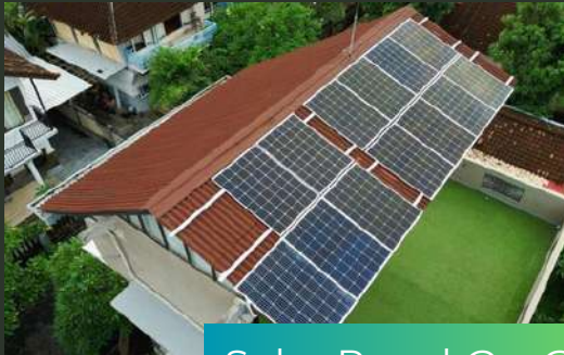
Solar Panel On-Grid
