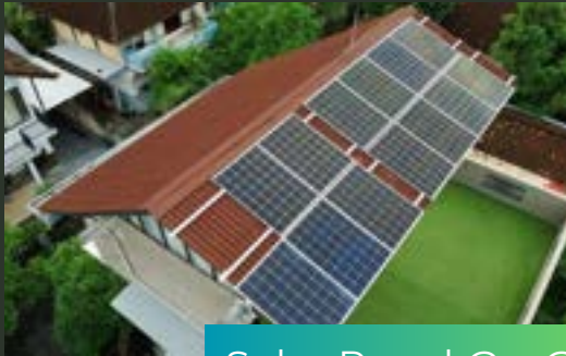
Solar Panel On-Grid
